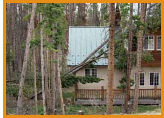
Figure 21: During high winds, these lodgepole pine trees fell onto the house. Lodgepole pine is highly susceptible to windthrow. Photo: CSFS
